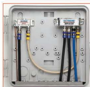
Unique Data-Plus™ Splitter Installation
