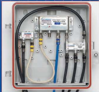
Infinity Premise VoIP/Modem Installation
