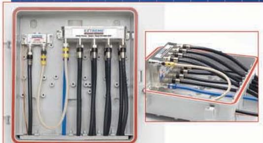
Infinity Premise VoIP/Modem Installation
